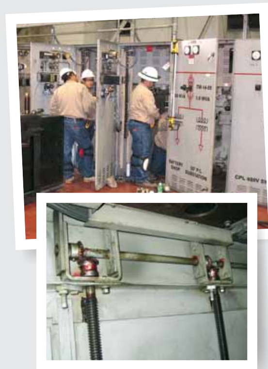
Above: WES's manufacturing capabilities and extensive parts inventory were on full display when it rebuilt all cubicles for more than a dozen Magne-Blast circuit breakers for a U.S. steel manufacturer. Left: GE Magne-Blast AM 13.8-750-2H 2000-amp with VCP-WR element air-magnetic circuit breaker that has been vacuum retrofitted.
